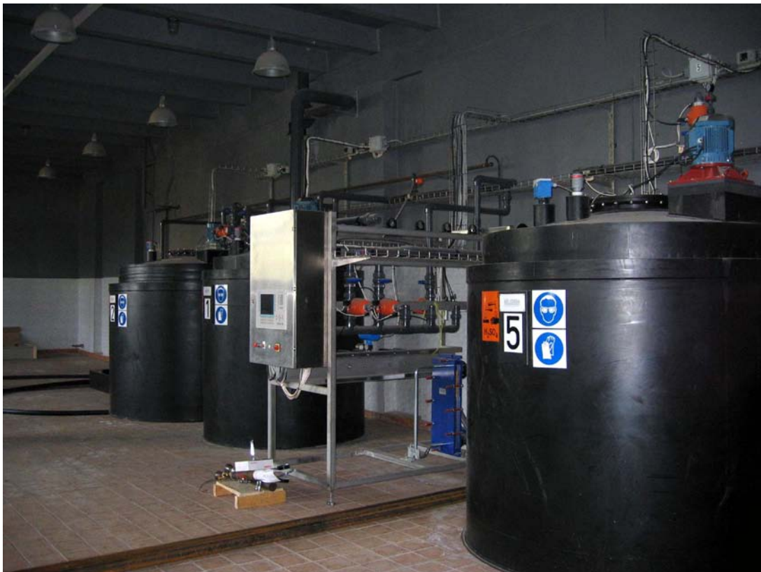
Acid mixing system
